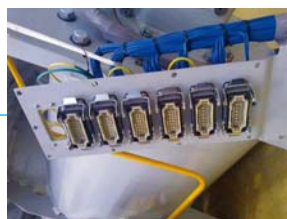
■ High - tension switch cabinet
