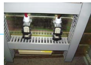
■ Box - type substation
