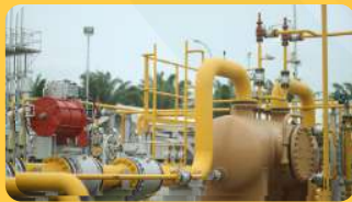
Natural Gas Pipeline 75 MMSCFD
