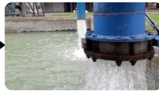
Water Treatment Plant 250 m 3 / hour
