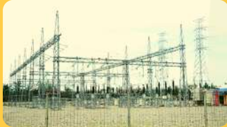
Electricity 150 KV/ 60 MVA
