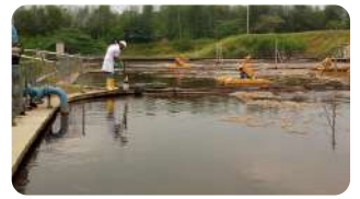
Waste Water Treatment Plant 250 m 3 / hour
