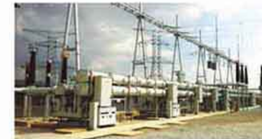
220kV Yun Nan-Jinzhong GIS Substation
