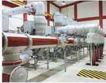
Mexico CFE 1521 115kV GIS Substation
