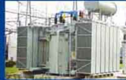
BKS-60000/35 Oil Immersed Shunt Reactor Running in Anhui Electric Power Company
