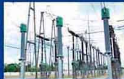
LVQB-550 SF6 Current Transformer Running in Philippines State Power Corporation
