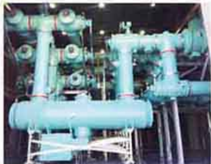
Mexico CFE 420kV GIS SE 1701 Substation Chimalpa Dos
