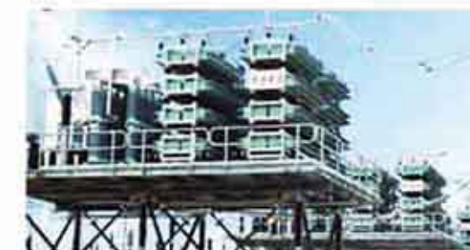
Guangxi Hezhou 500kV Substation Serial Compensation Capacitor Bank
