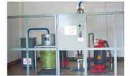
Peterson Coil Complete with Automatic Tuning and Fault Line Selection for indoor
