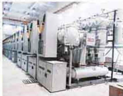
India TANTRANSCO Guindy 230 110kV GIS Substation Project
