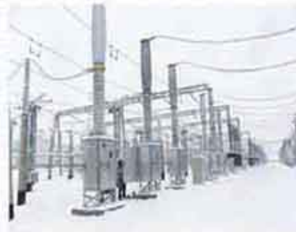
Belarus 330kV Substation Project
