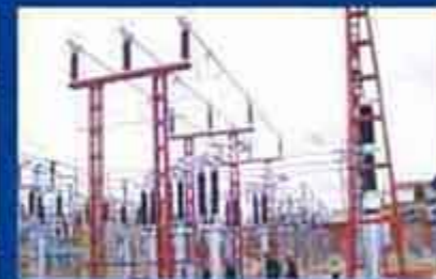
LW36-72.5 SF6 Circuit Breaker Running in Madagascar
