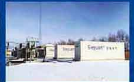
33kV STATCOM Project in Jilin Wind Farm
