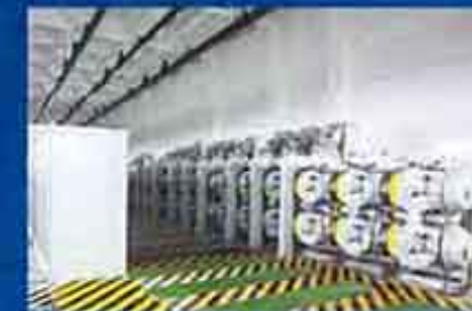
Beijing Future City Station 145kV GIS Substation
