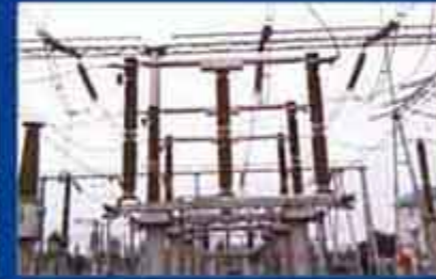
GW7B-252 Disconnecter Running in Ningxia Electric Power Company
