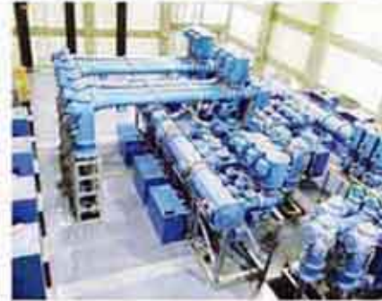
Mexico CFE 237LT 1313 252kV GIS Substation
