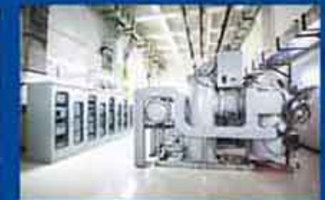
Bewu Village 145kV GIS Substation
