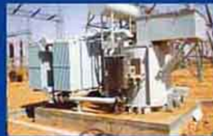
BKS-15000/11 Oil Immersed Shunt Reactor Export to Sudan State Power Corporation
