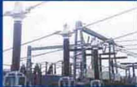
66-420KV Instrument Transformer Run in National Grid Electricity Transmission PLC
