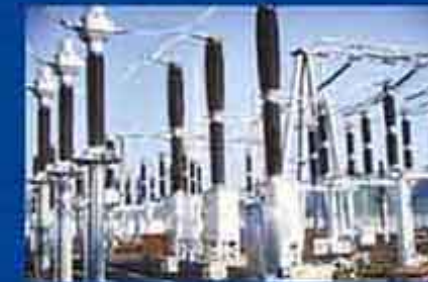
220kV Shihezi Oasis Substation
