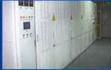
STATCOM Running at Shanghai Expo Mengzi Substation
