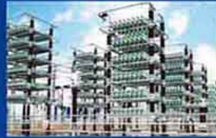
TBB525-301824/524AQW Shunt Capacitor and Installation Running at Yunnan-Guangzhou UHV Converter Station
