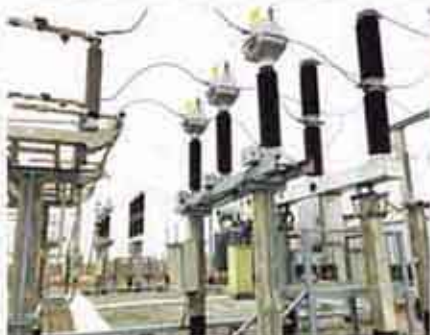
Uzbekistan Modernization of south-west transmission network (stagell) within 220kV & 110kV Talimarjan Transmission Project
