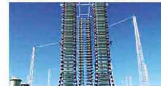
ShanghaiMiao-LinYi ± 800kV HVDC Transmission Project
