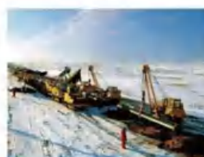
Uzbekistan section of Central Asia gas pipeline
