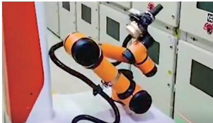
High-voltage distribution cabinet operation
